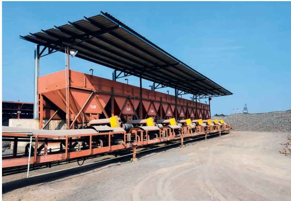
▲ Automated raw material hopper: the weighing system measures out the required quantity of waste materials for the specific batch.
